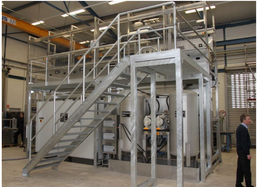
The HFE system on the manufacturer's premises ready for test operation and acceptance by the operator.
