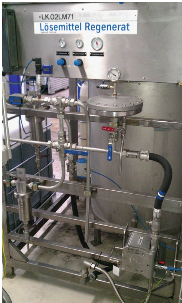
Integrated double diaphragm pump in use by a supplier to the automotive industry.
