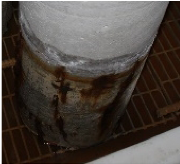
Fig. 5 External signs of corrosion on day 11 for specimen NN-R-1
