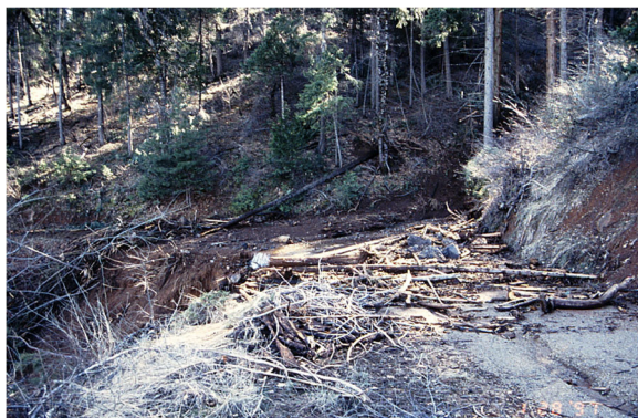
Fig. 5 The flow path of the Pilot Ridge debris flow where it crossed Forest Road 1566. Note the levees of soil and transported trees left on the road and the undermining of the roadbed by the debris flow's passage
