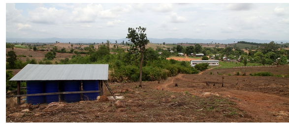
Fig. 1 Three water storage tanks were installed by the study team covered by a corrugate iron roof, which are a part of the improved water supply system provided as a community incentive to the village in the background
