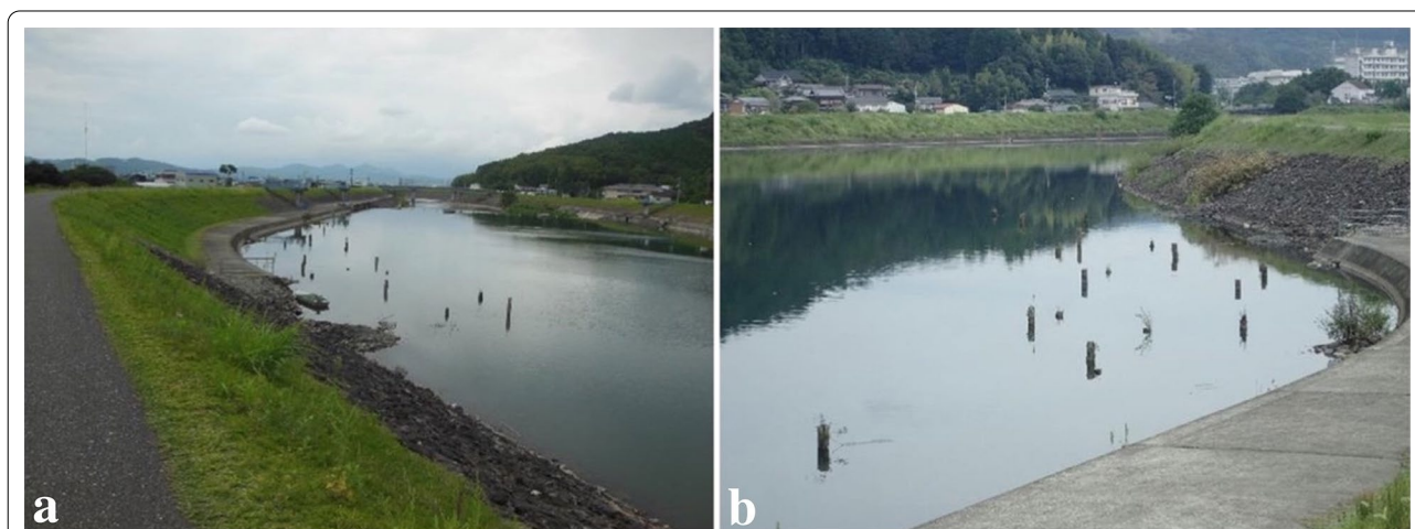
Fig. 1 A full view of river groynes using logs in the Kokubu River: a from the upstream side, b from the downstream side
