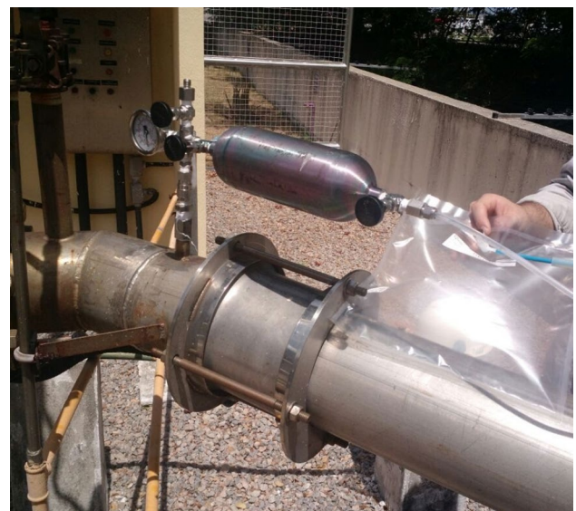
Fig. 3 Biogas collection performed at the Baldo STP on 24/10/2017
