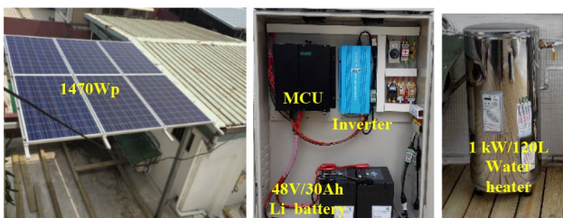
Fig. 4 HyPV D5 installed in an apartment (Taipei)
