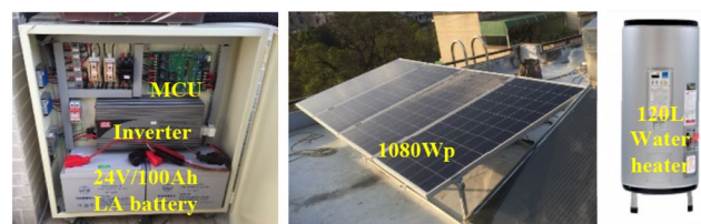
Fig. 6 HyPV D11 installed in a house (Chia-Yi)
