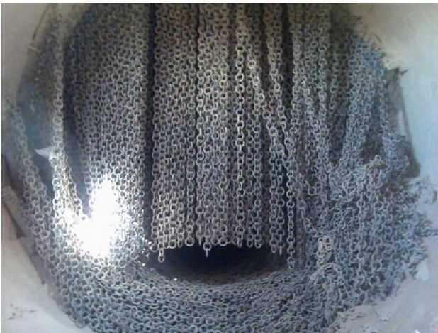
Fig. 2 A real image of chains curtain inside rotary cement kiln at Kufa cement plant . Courtesy of Kufa cement plant (image no. CK-005)
