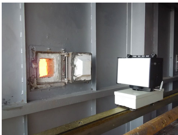
Fig. 4 Temperature measurement process for ethylene cracking furnace tube
