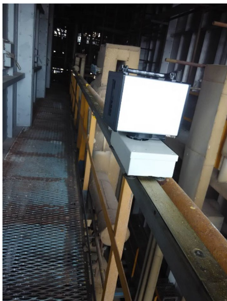
Fig. 3 Real temperature measurement system
