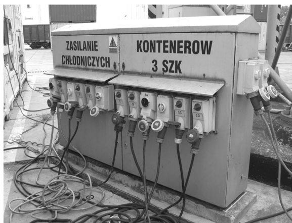
Fig. 1 Station to plug refrigerated containers in Szczecin seaport
