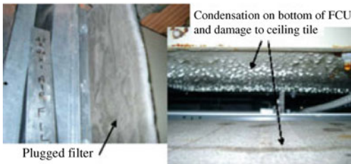
Plugged filter causing condensation on bottom of fan coil unit and damage to insulation coil resulting in poor air flow [Martha Hewett, MNCEE]
