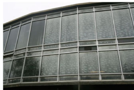
Failed window film treatment
