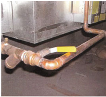
Hot water valve motion impeded by piping layout [EMC no date (a)]
