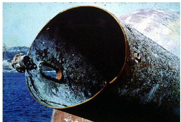
Fig. 2 Fatigue crack propagated part way round the insert and then the brace
