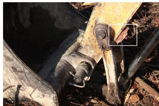
Fig. 18 Fillet weld cold laps are usually located on the bottom side of the weld. Here, an excavator has been poorly repaired in the field, and due to the generation of a cold weld, the structure failed soon after
