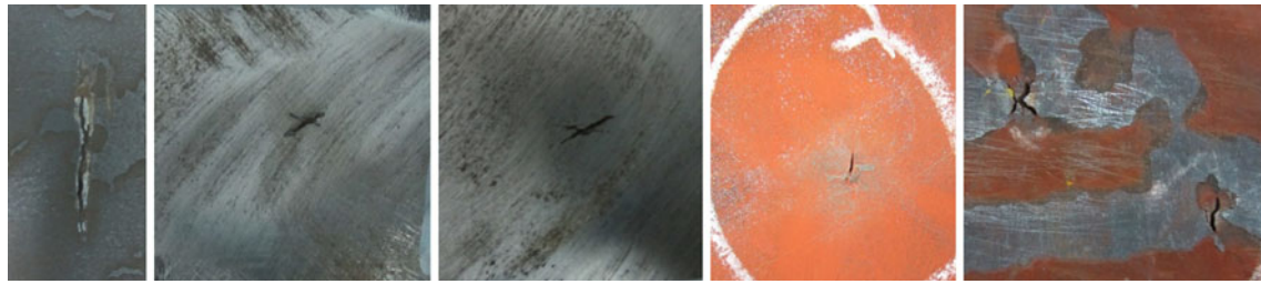
Fig. 1 Crack photos observed on the extrados portion of the bend
