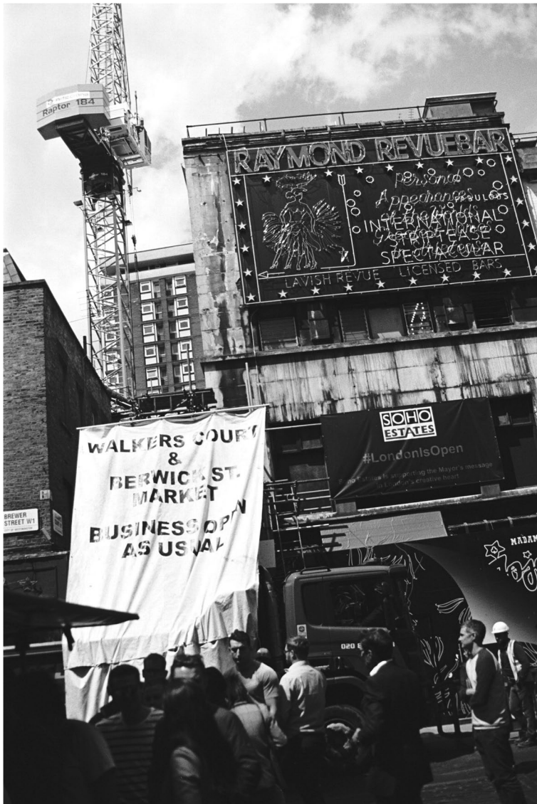
Fig. 1 The former cabaret and burlesque night club Madame Jojo's is being renovated to accommodate a more affluent clientele (photo by R. Stam)
