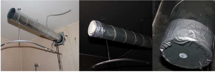
Figure 2. The three ventilation duct configurations used in the experiments—Open, Normal and Closed (left to right).
