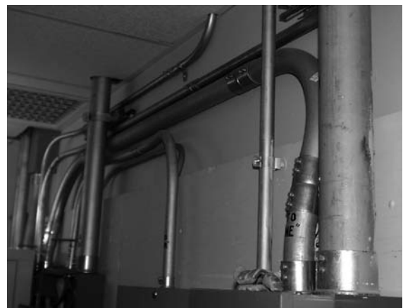
Fig. 10 If rack cabinets are concealed in equipment closets, the electrical troughs and/or pipes coming down from the ceiling or up from the floor can be surface-mounted on the back wall without concern about their appearance. This can save new and renovation costs throughout the lifetime of the procedure room. Reprinted with permission of Medical Physics Publishing [7]
