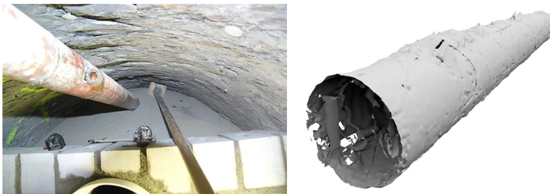
Fig. 5 Left Granular buffer emplacement using an auger system, right 3D image of the microtunnel test section before installation for volume calculation (Gaus et al. 2014)
