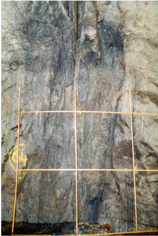
Fig. 8 Photograph of fault F64 at Tm 4,670, including a 1 m-grid scale
