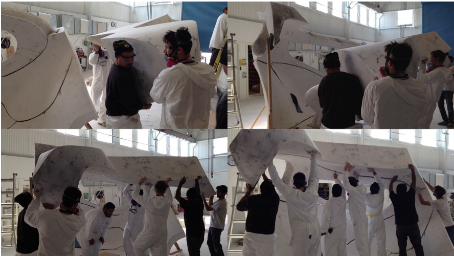
Fig. 21 The Cyclopean parts of the pavilion are light enough to be manually lifted into place
