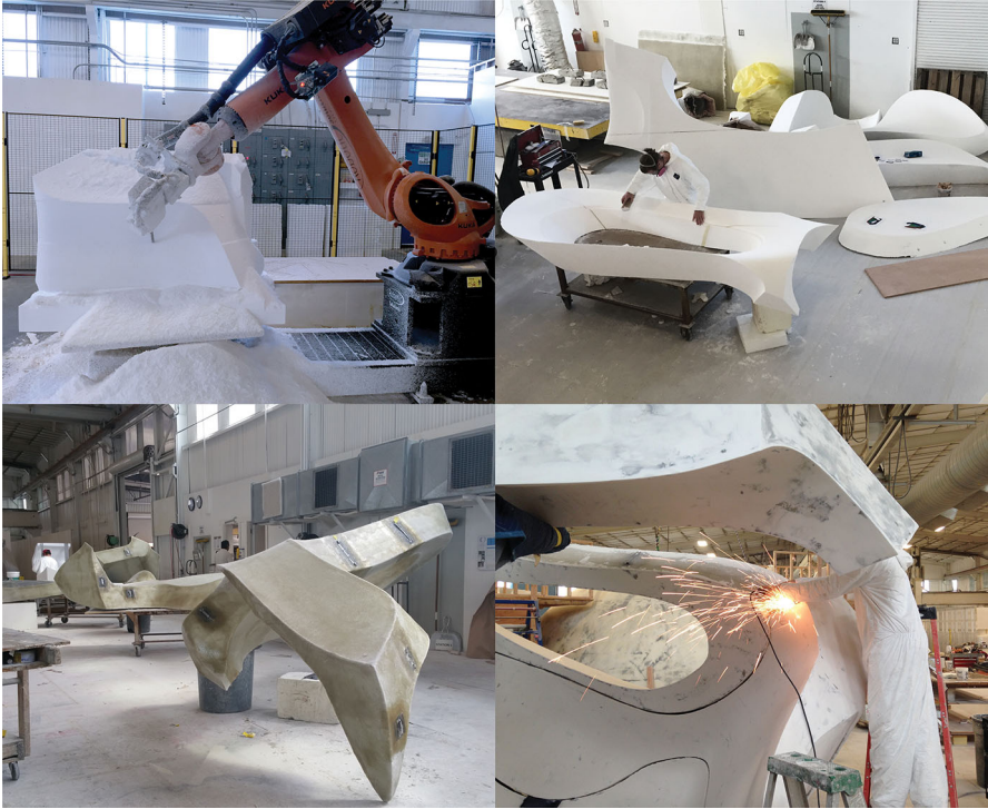
Fig. 20 The pavilion is made from foam parts cut by robots and other large CNC cutting tools. The parts are wrapped in a 2 mm thick layer of glass-fiber reinforced plastic
