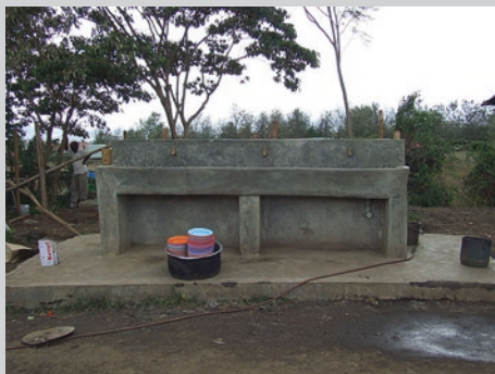
Image 3.2 Gray water reuse facility at secondary school. (Credit: The Sustainable Sanitation Alliance Secretariat/CC BY)
