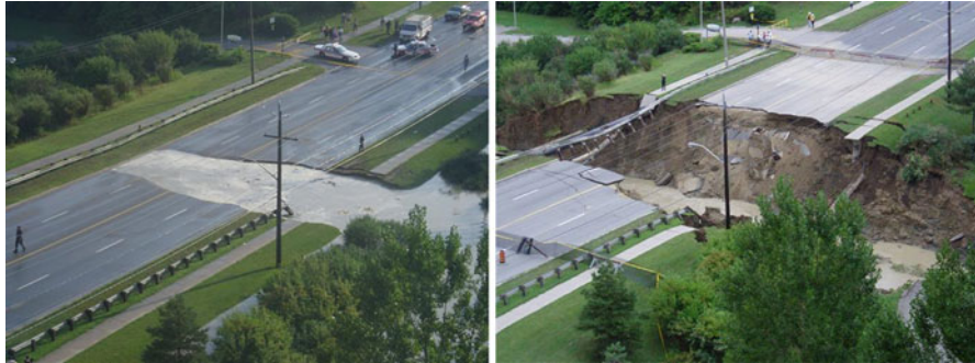
Fig. 1.11 A caved-in culvert at Finch and Sentinel in the north of the city during the 2005 flooding
