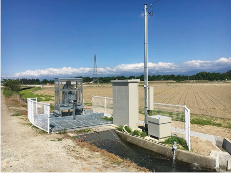
Fig. 4.2 Small hydroelectric power generation using agricultural water. (Courtesy: Imagineer Co., Ltd.)
