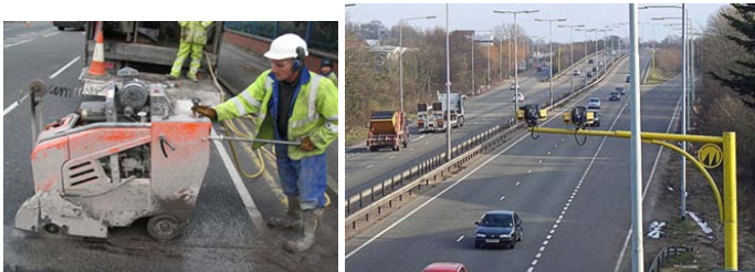
Fig. 1. Left: Installation of intrusive loops. Right: Computer Vision sensors.
