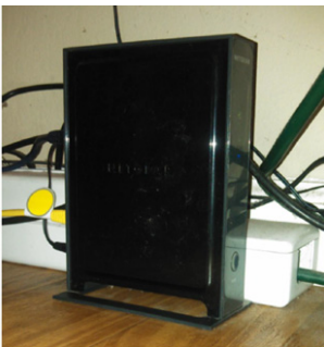
Fig. 8. Router in open air with vertical positioning
