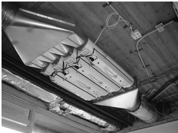
Fig. 18.1 In-duct UVGI system retrofit into an existing ventilation duct. System consists of four modular axial UV lamp fixtures. Photo courtesy of Virobuster Electronic Air Sterilization, Marthalaan, The Netherlands
