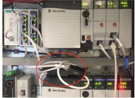
Fig. 7. Raspberry Pi3 connected between PLCs.
