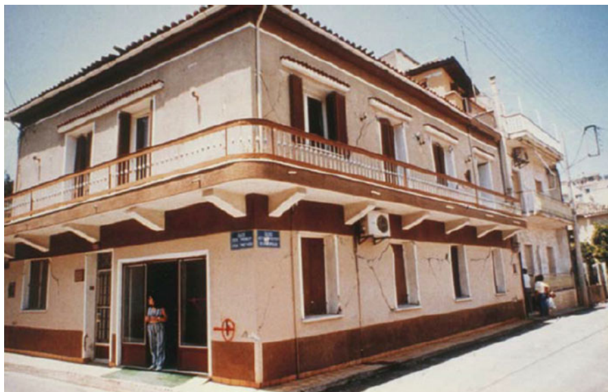
Fig. 16.8 Unreinforced masonry with RC floors, grade of damage 3, in Greece 1995 (Grünthal 1998, EMS-98 scale)
