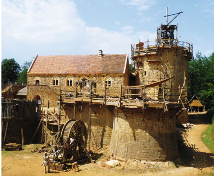
View on the building site of the castle of Guédelon, France, from the south-west (Guédelon, 2012).
