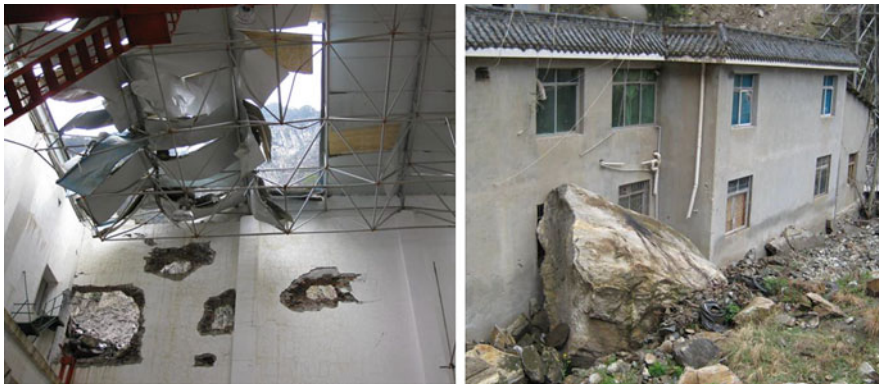
Fig. 20.4 Infill wall and roof of powerhouse punctured by high-velocity rocks ( left ) and wall damage of building of Shapai power plant by large rock ( right ) caused by 2008 Wenchuan earthquake
