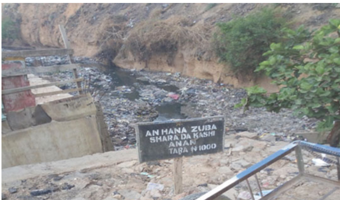
Fig. 8 Indiscriminate dumping of waste along drainage in the study area. (Source: Field Survey 2019)
