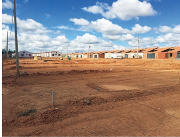
Fig. 5.20 Social housing in construction in Montes Claros in 2015. (Reproduced with permission from Bolay)
