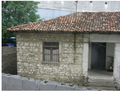
Fig. 7.10 Horizontal timber embedded in load-bearing wall masonry ( hatil construction). Wooden boards, when tied around the facade-side wall junctions aid in reducing the occurrence of corner wedge failures. These horizontal boards accept lateral loads during seismic shaking (Dogangün et al. 2006). Elbasan, Albania (Photo M. Kázmér, #8769)
