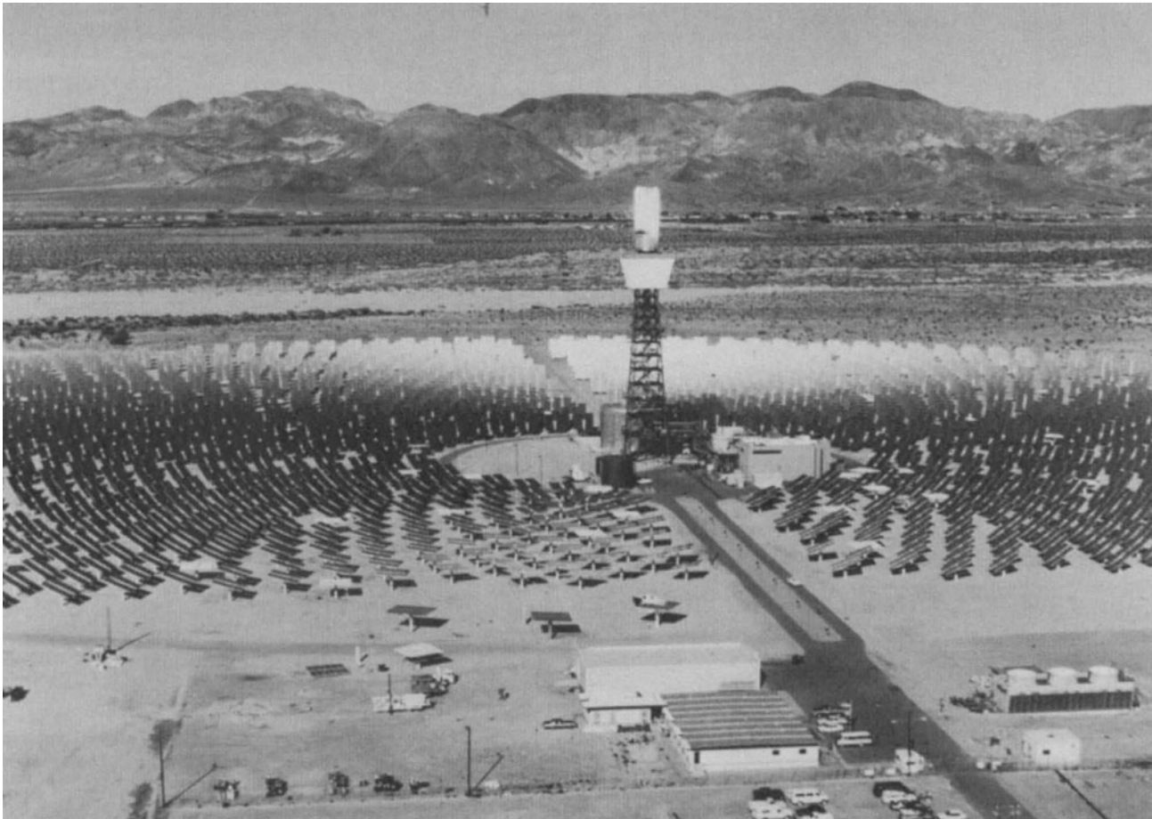
Fig. 16. Panoramic view of the world's largest solar thermal electric power plant, located on the Mojave Desert, near Daggett, California. The 10 megawatt (electric) facility commenced operation in 1982 and achieved design capacity in 1984. The collector tower (receiver upon which solar energy is reflected) is located atop a 300-foot (91-meter) tower. The north field of heliostats (mirrors kept in synchronism with the movement of the sun), 1240 in number, is shown in background; the south field (578 heliostats) is shown in foreground. Operating facilities, turbine generators, and storage tank are shown in circular middle section under the tower. The facility is operated by Southern California Edison and the Los Angeles Department of Water and Power, in conjunction with the U.S. Department of Energy and the California Energy Commission.
