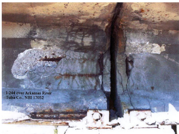
Fig. 1 Damage in the end region of an AASHTO bridge girder.
