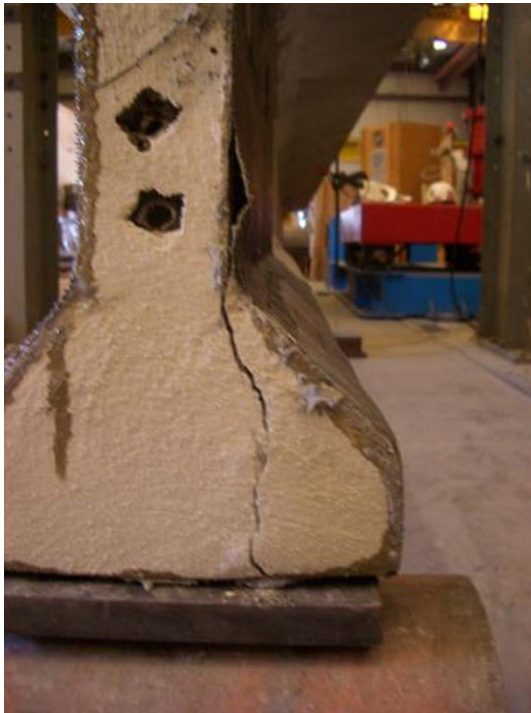
Fig. 8 Premature crack on beam 1 end A .
