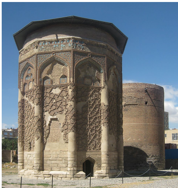
Fig. 1 The Blue Tomb (Gunbad-i-Qabud), built in A.D. 1196–97 in Maragha, western Iran. Photograph for Figure was taken by M. Ghari (Teheran)
