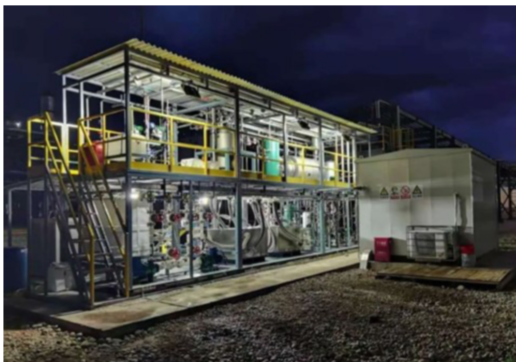
Fig. 12. The demonstration system of \text{CO}_2 electrolysis for syngas production [Reprinted from (Carbon Energy Technology Co. LTD, 2020)].
