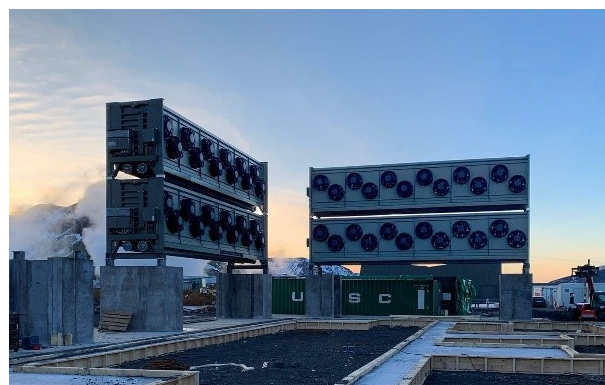
Fig. 3. Orca plant from Climeworks [(©climeworks, 2022), used with permission].
