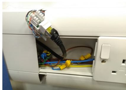
(b) The prototype attack device in situ inside service trunking on an office wall.
